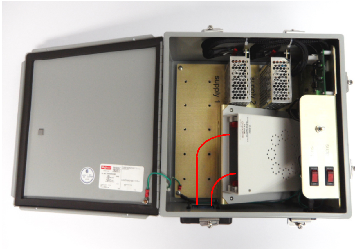
Figure 5. RF & Optical Cable Routing Within EZLink
